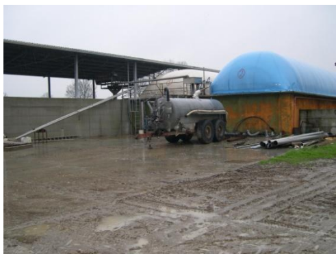
Biogas digestors, Photo: CRPA
